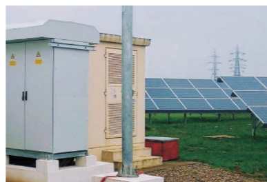
Energy Storage Cabinet
